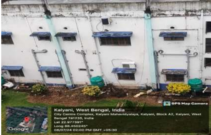
Rain- Water Harvesting/ re-use Project
